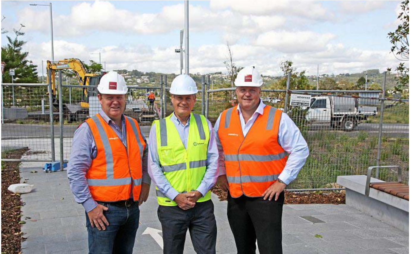
Evans Long directors Dirk Long, left, and Matt Evans, right, with SunCentral CEO John Knaggs on site at Maroochydore CBD.
